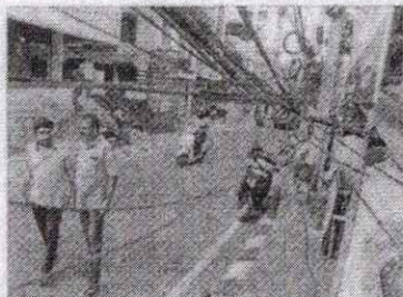
Low-lying cables at Layam Road where Sabu and his wife Sindhu met with an accident and escaped with minor injuries | AISHWARYA PRABHAKARAN
